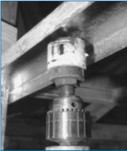
Pre-punched holes are provided in LSF studs and joists, but site-cut holes can be made with hollow core drill bits as shown here for a custom track hole.
